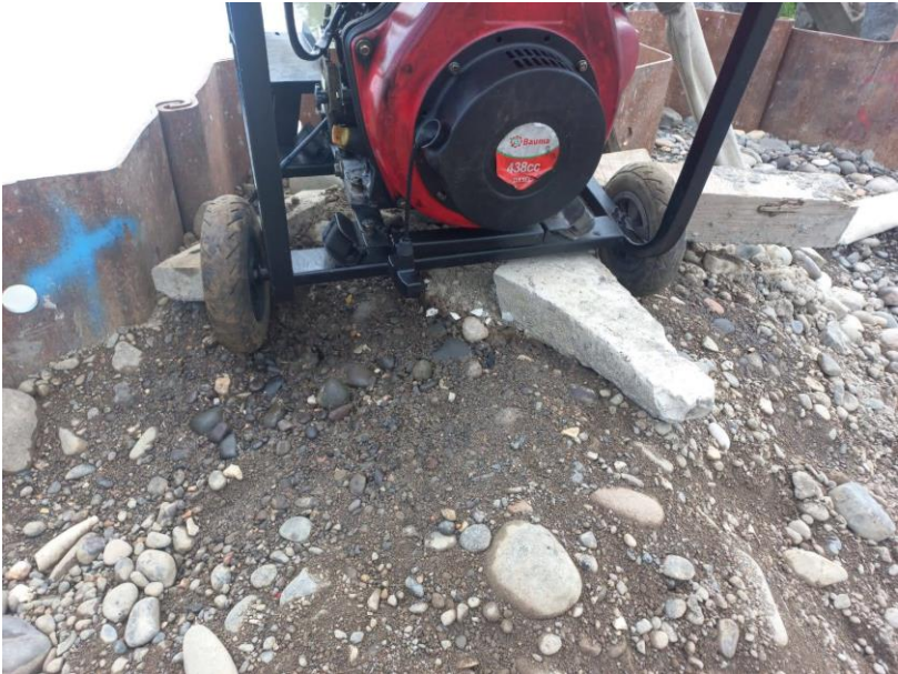
Oil spillage on site
