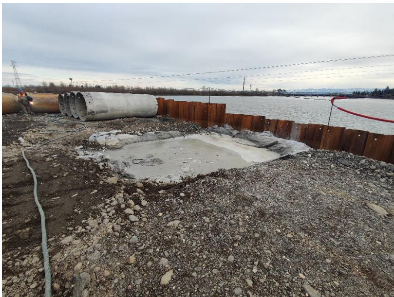
Sediment trap for the cement and excess water in the peninsula
