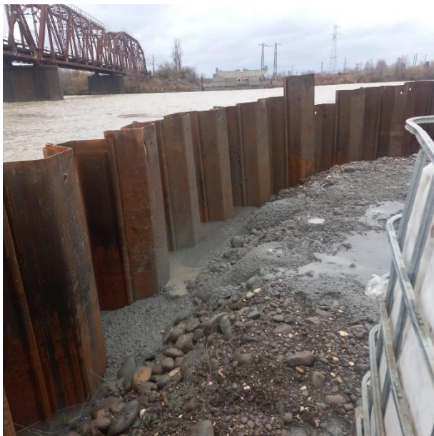
Cement Spill into the River from the Peninsula
